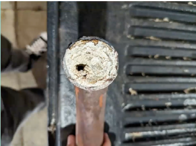
Figure 1: The ruptured boiler tube, filled with calcium deposits.
